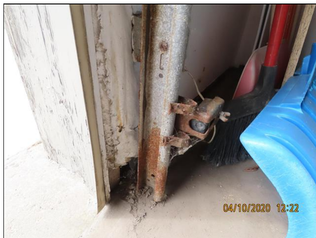
3.2 Item 2(Picture) localized moisture near overhead garage doors
