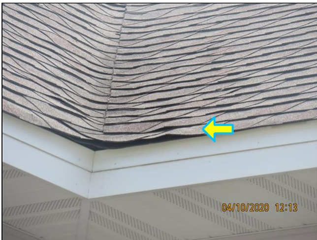
1.0 Item 8(Picture) lifted flashing rear of home
