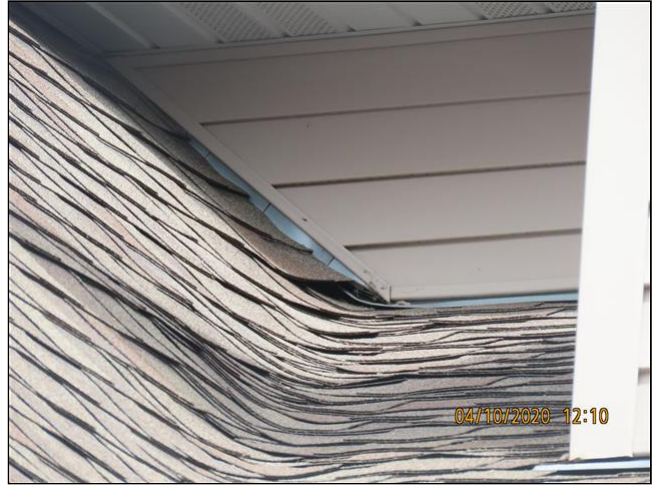
1.0 Item 5(Picture) lifted shingle, front of home
