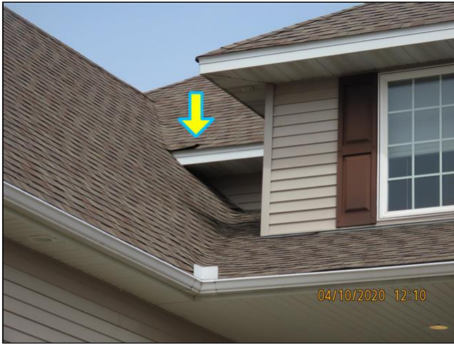
1.0 Item 4(Picture) lifted shingle, front of home
