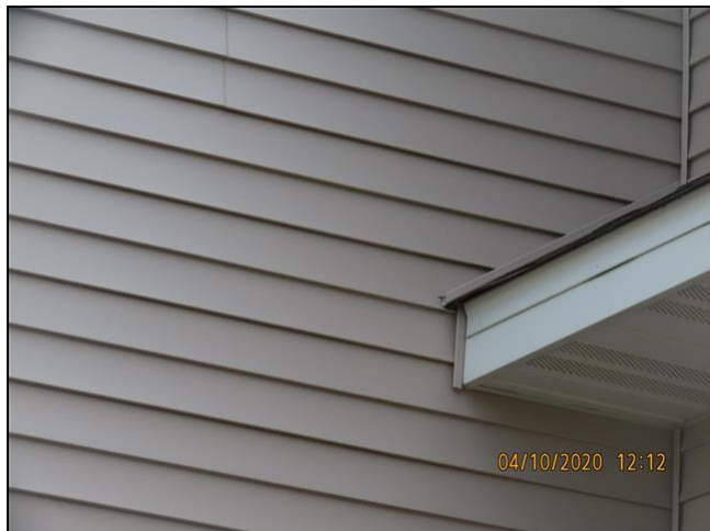
1.2 Item 1(Picture) missing flashing, rear of home
