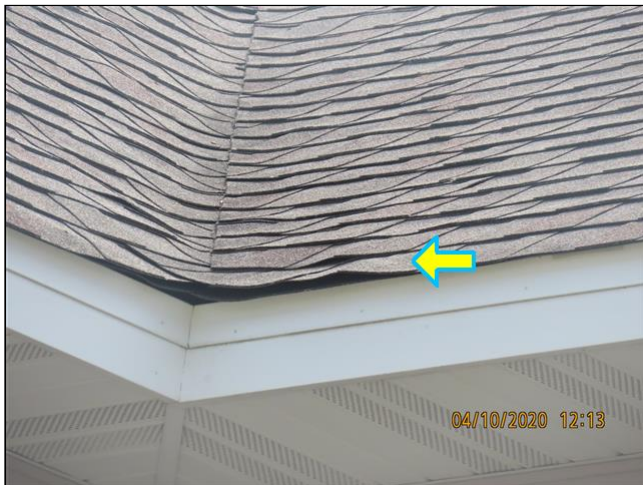
1.0 Item 8(Picture) lifted flashing rear of home
