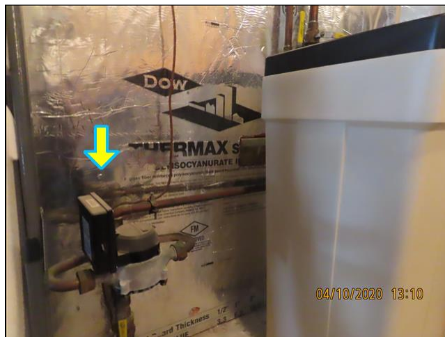
main water supply
