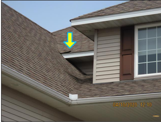
1.0 Item 4(Picture) lifted shingle, front of home
