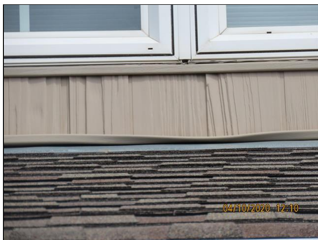
2.3 Item 1(Picture) damaged flashing, front of home
