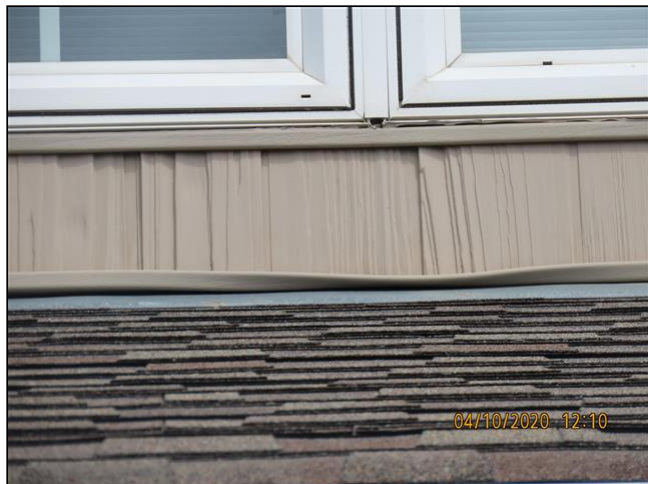
2.3 Item 1(Picture) damaged flashing, front of home
