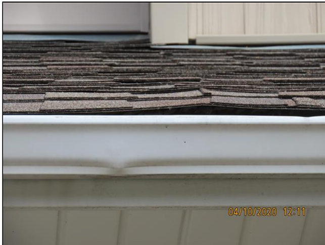
1.0 Item 6(Picture) lifted shingle, front of home
