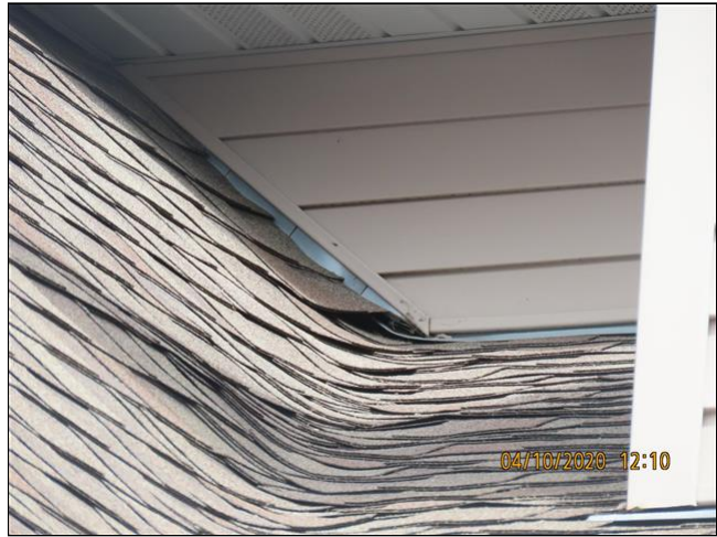
1.0 Item 5(Picture) lifted shingle, front of home
