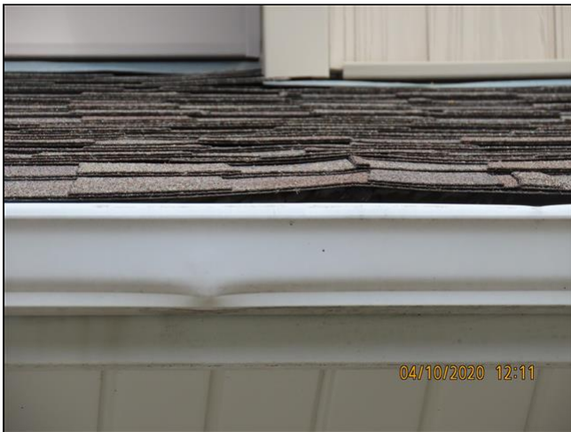
1.0 Item 6(Picture) lifted shingle, front of home
