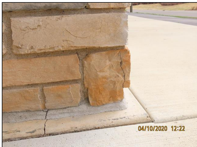
2.1 Item 1(Picture) front of home, near garage door
